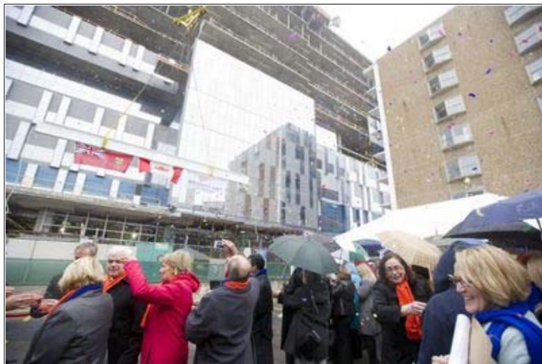
Bridgepoint Health half way to completion. The final steel beam is hoisted into place at Bridgepoint Health during a topping off ceremony for the new 10-storey building, which will serve patients with complex, chronic disease and disability in south Riverdale. (Oct. 26, 2011) Staff photo/NICK PERRY
